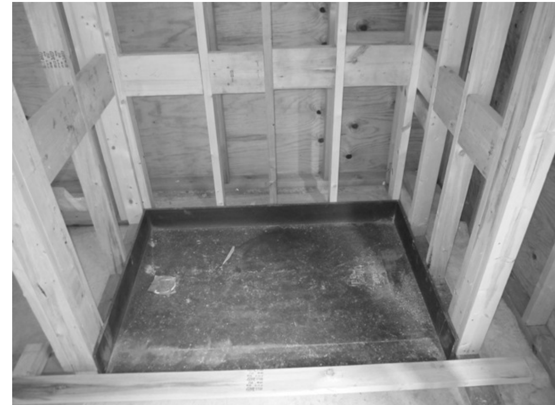
NOTE: ADD BLOCKING AS REQUIRED FOR HANDI CAP GRAB BARS IN ALL MODELS. VERIFY LOCATIONS OF BLOCKING BEFORE START OF CONSTRUCTION
