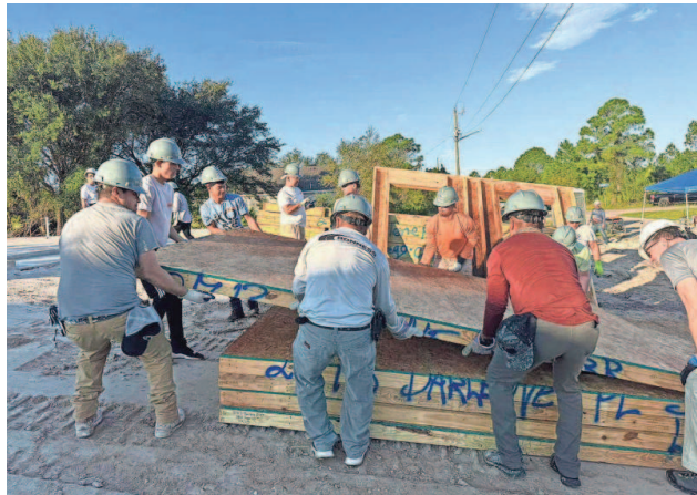
On Oct. 26, Habitat volunteers, sponsors and fellow veterans assisted Osvaldo in building and raising the exterior walls of his future home in Lehigh Acres.
